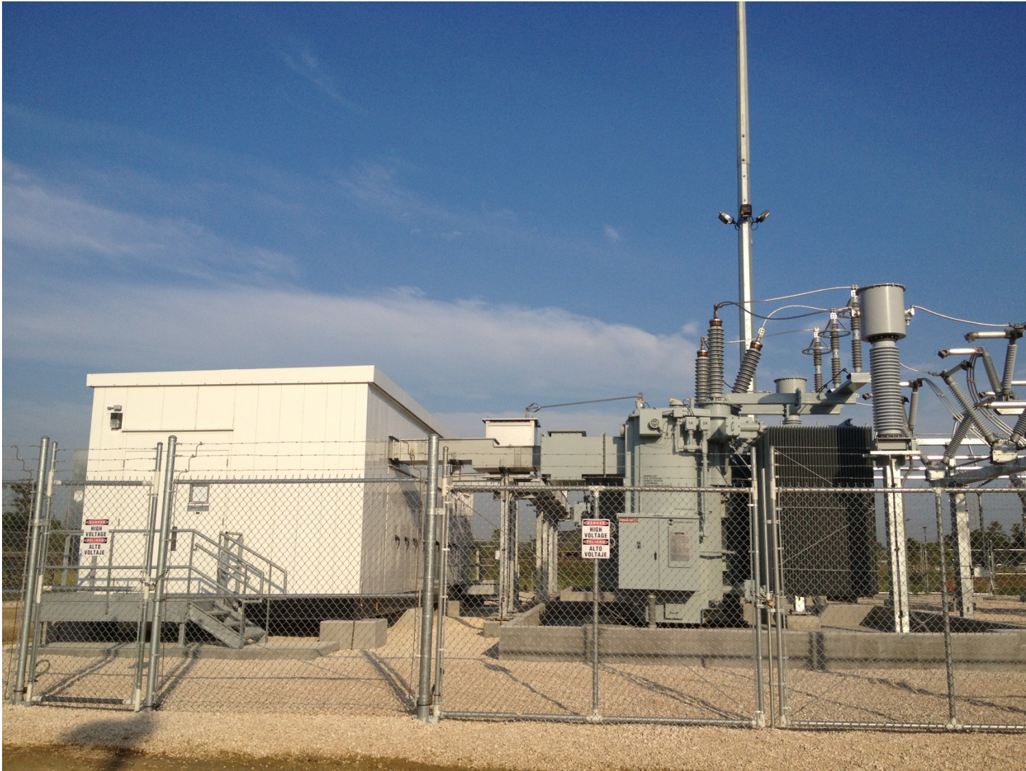
Typical 138 kV Substation
